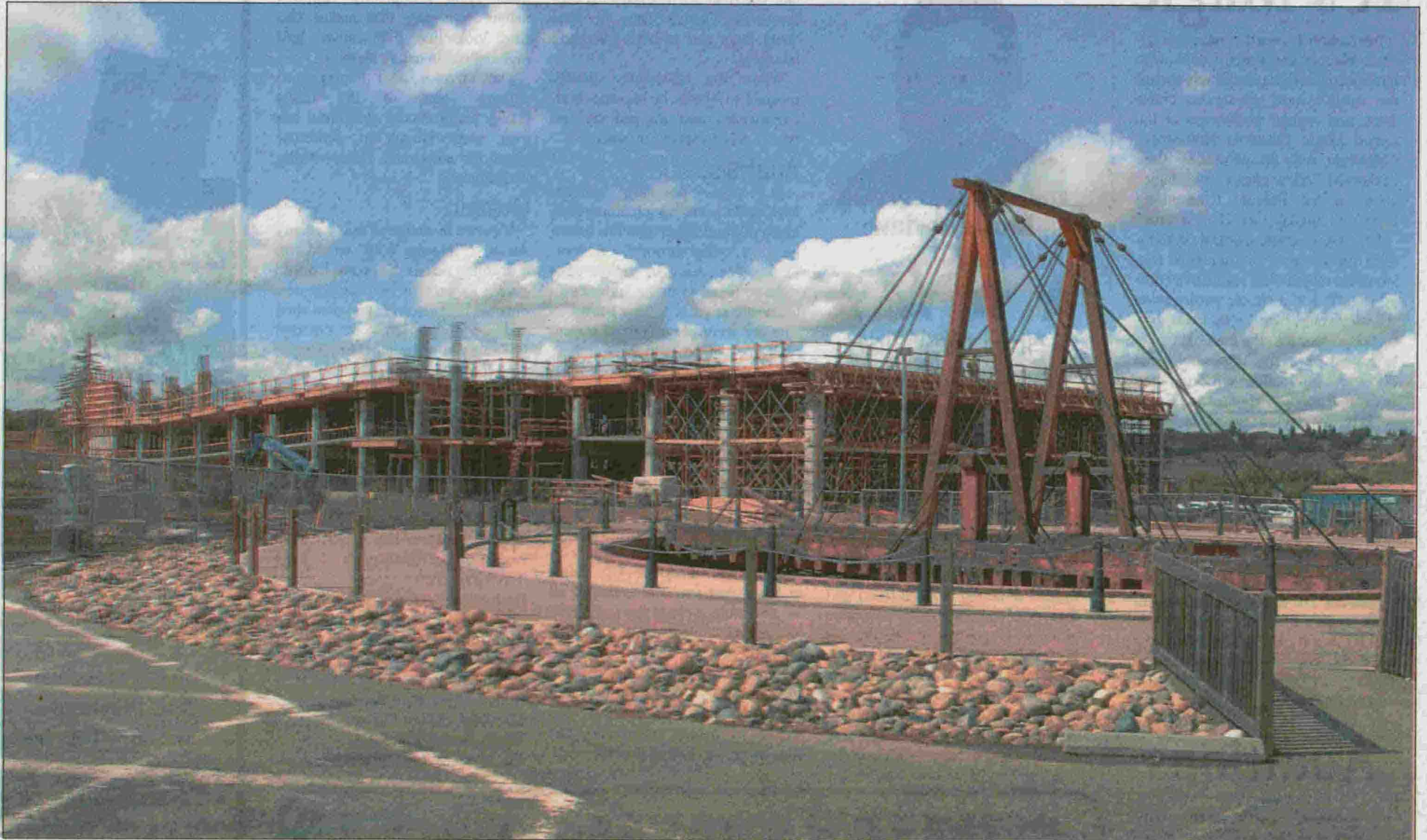
SEEN THROUGH THE ROUNDHOUSE GIRDERS, the 4-story parking garage is scheduled to open in 2008 next to the light rail station.
